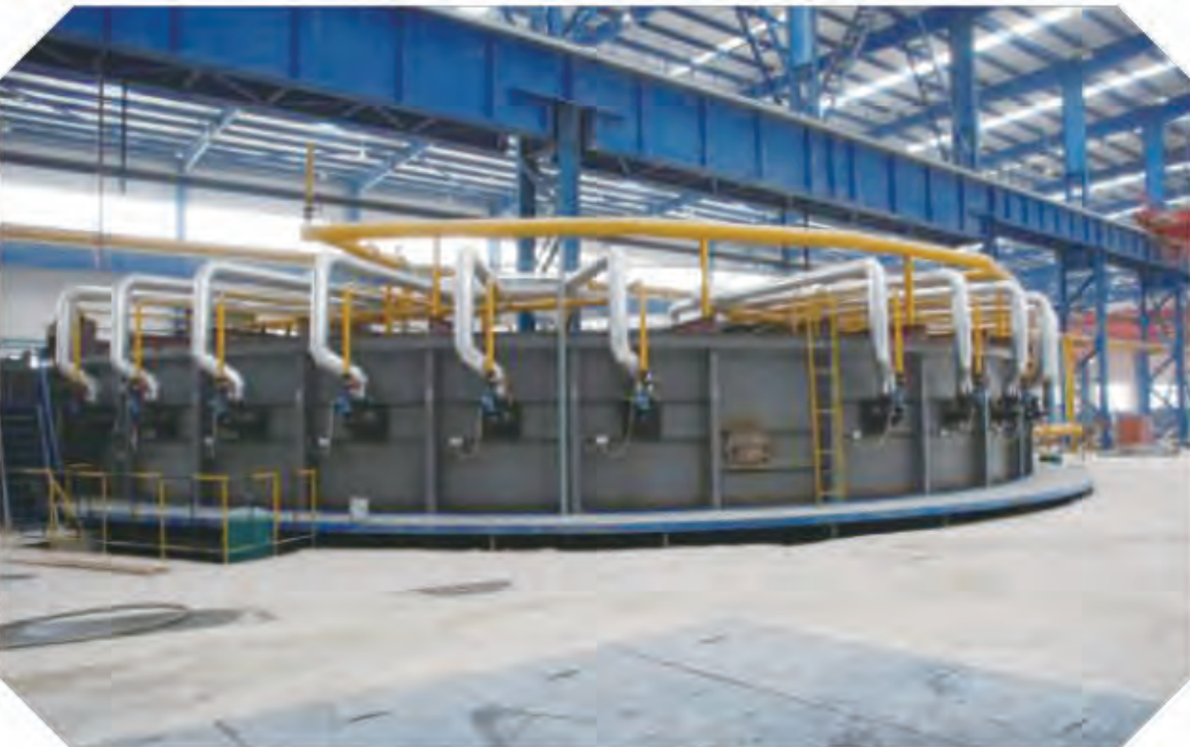
18 米环形加热炉 18m Rotary heating furnace
