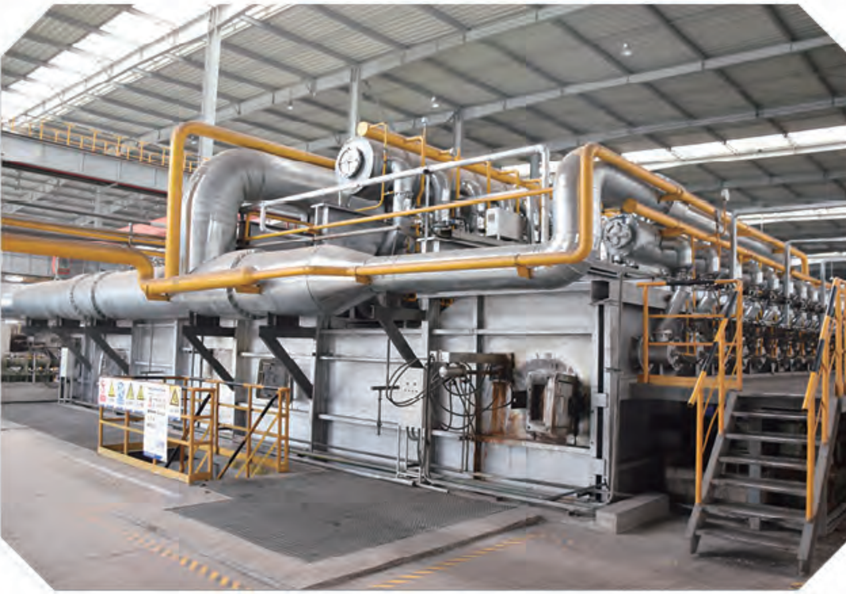
回火炉 Tempering furnace
