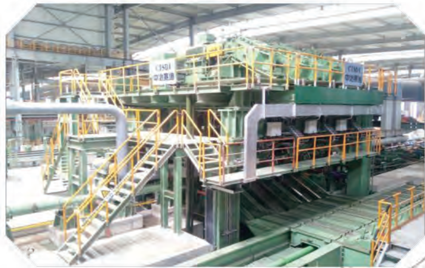
五机架三辊连轧机 5 stands 3-roll continuous rolling mill
