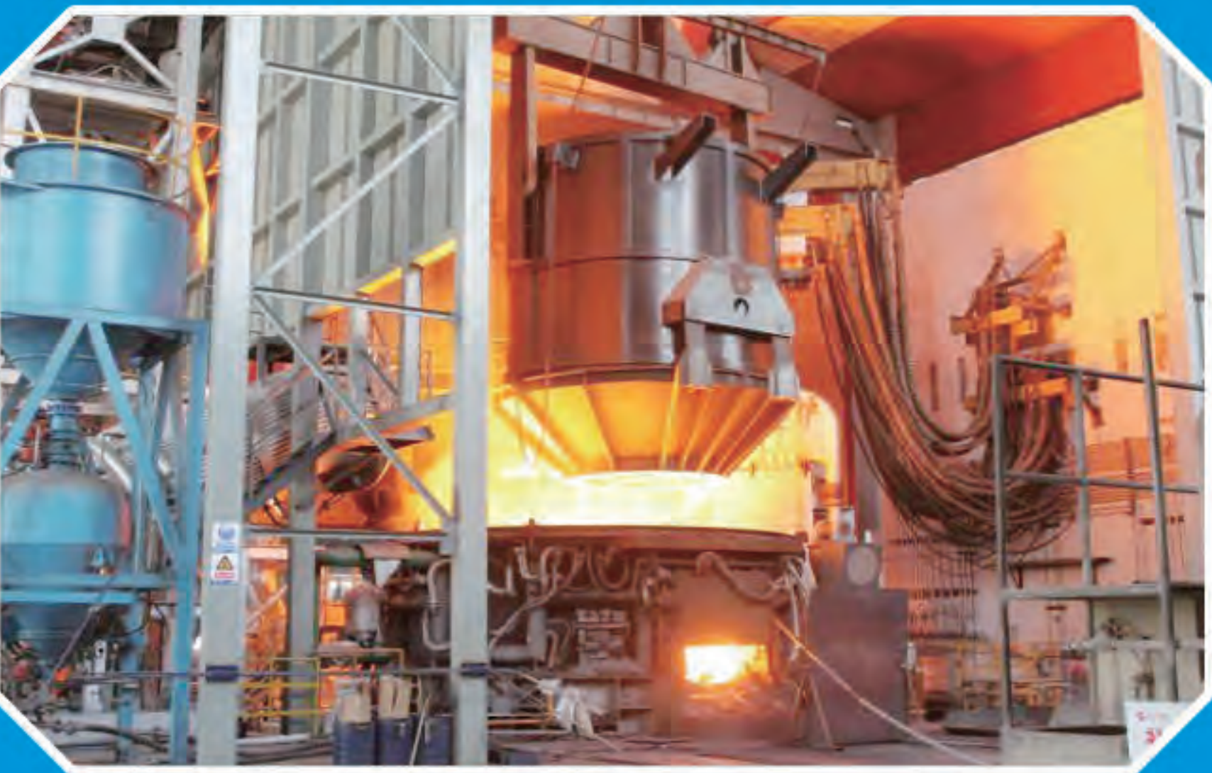
超高功率电弧炉 Ultra-high power electric arc furnace
